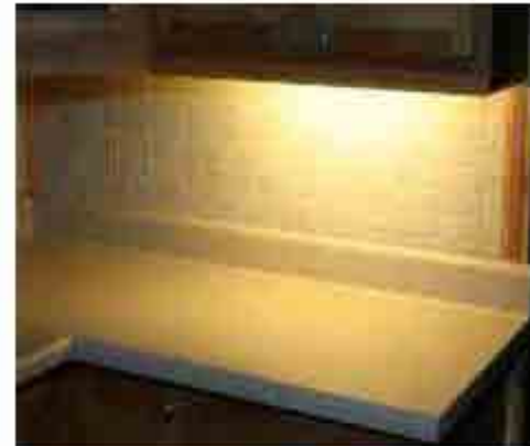
14 watt T5 linear fixture Average illuminance: 405 lux Minimum illuminance: 128 lux Meets recommendation for critical tasks? Yes Uniformity on counter: 3:1
