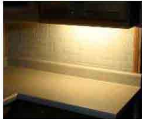
16 watt T4 linear fixture Average illuminance: 408 lux Minimum illuminance: 140 lux Meets recommendation for critical tasks? Yes Uniformity on counter: 3:1
